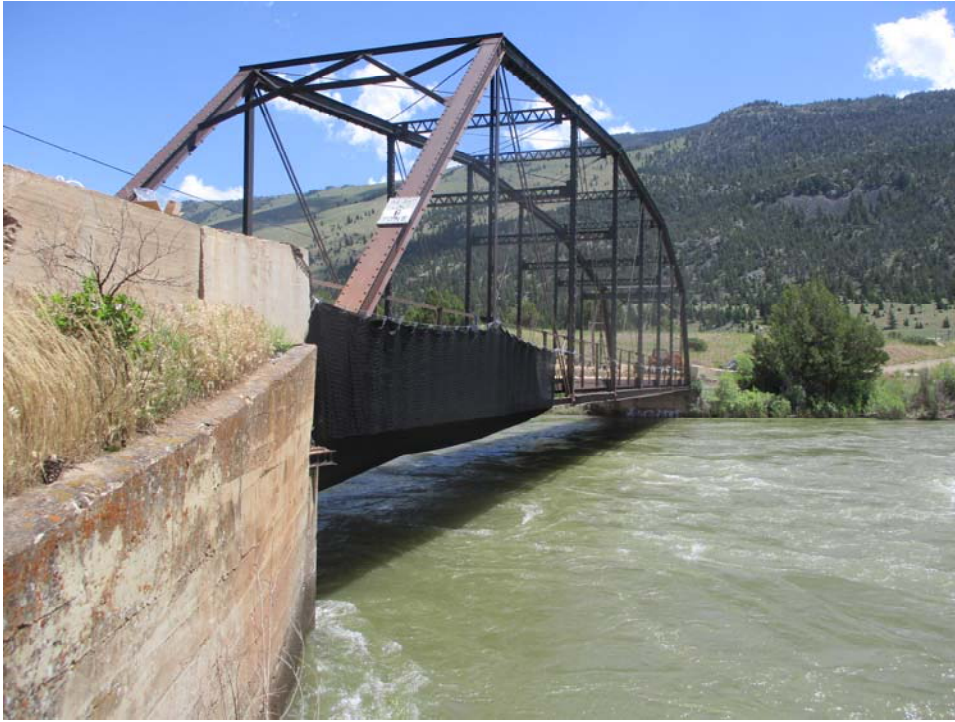
The debris shield installed beneath the first section of Carbella Bridge.
